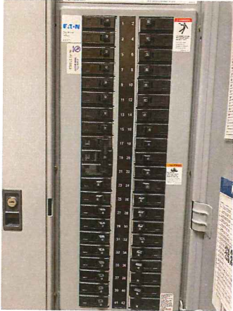
EXISTING ELECTRICAL PANEL 'L10' SECTION 1
